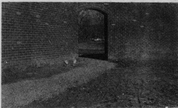
Despite the fact that there is an archway along the wall leading to the Moody Center, there is no paved entrance or exit. Weeks of wet weather prompted the placement of gravel on the path. There are, however, no plans to pave the messy walkway.
