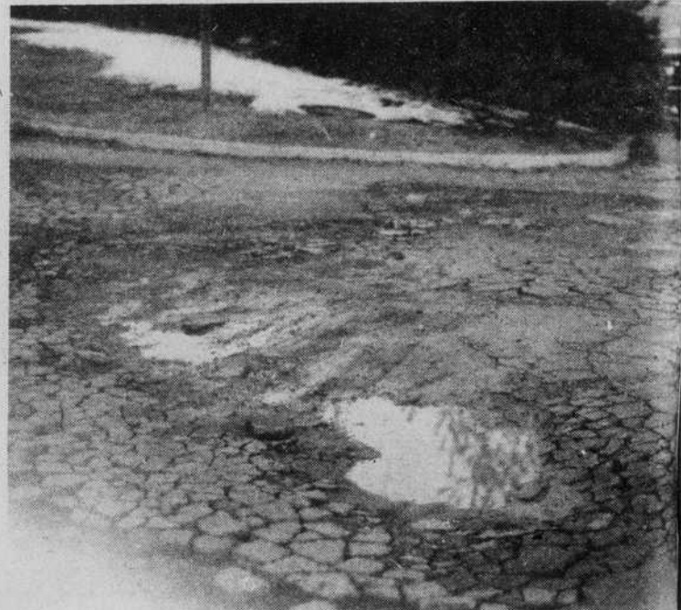
The potholes in front of the College apartments' entrance are a continental hazard to drivers. Photo by Debbie Lloyd
