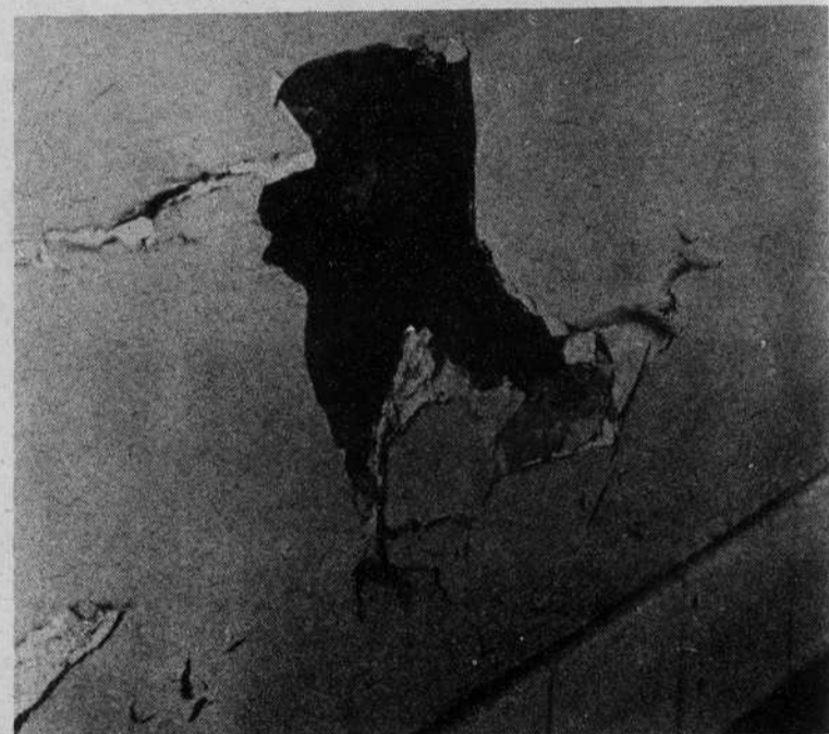
The inside wall of the swimming pool is cracked. The wall which has been left unrepaired for a month will apparently be left to deteriorate. Inside, the power plant is a maze of metal.
