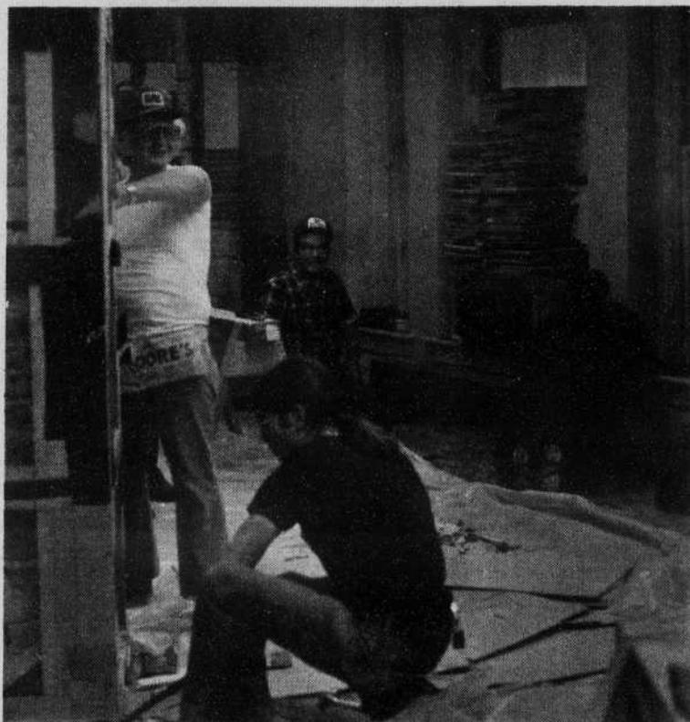
The old bookstore and switchboard office take on a new look as construction begins in Botetourt's basement. Construction workers are tearing out walls and surfaces and will build a larger switchboard office and an enclosed security office. Future plans include expanding the post office area. Photo by Anne Rood
